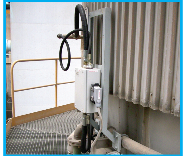
fig 3: lance box installed at the Calusco (ITA) cement plant
