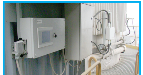
fig 4: master box installed at the Calusco (ITA) cement plant
